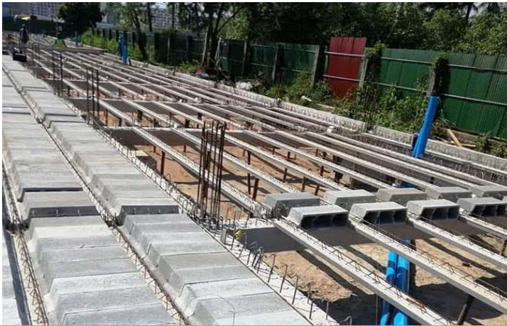
Girder and filler assembly A team of 10 workers can assemble 100m 2 per day
